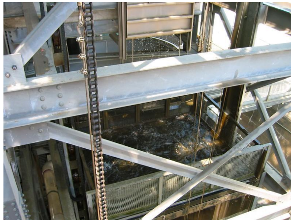
Fig. 3: Image of fish elevator transporting fish to higher waters (Cooper, 2012).
